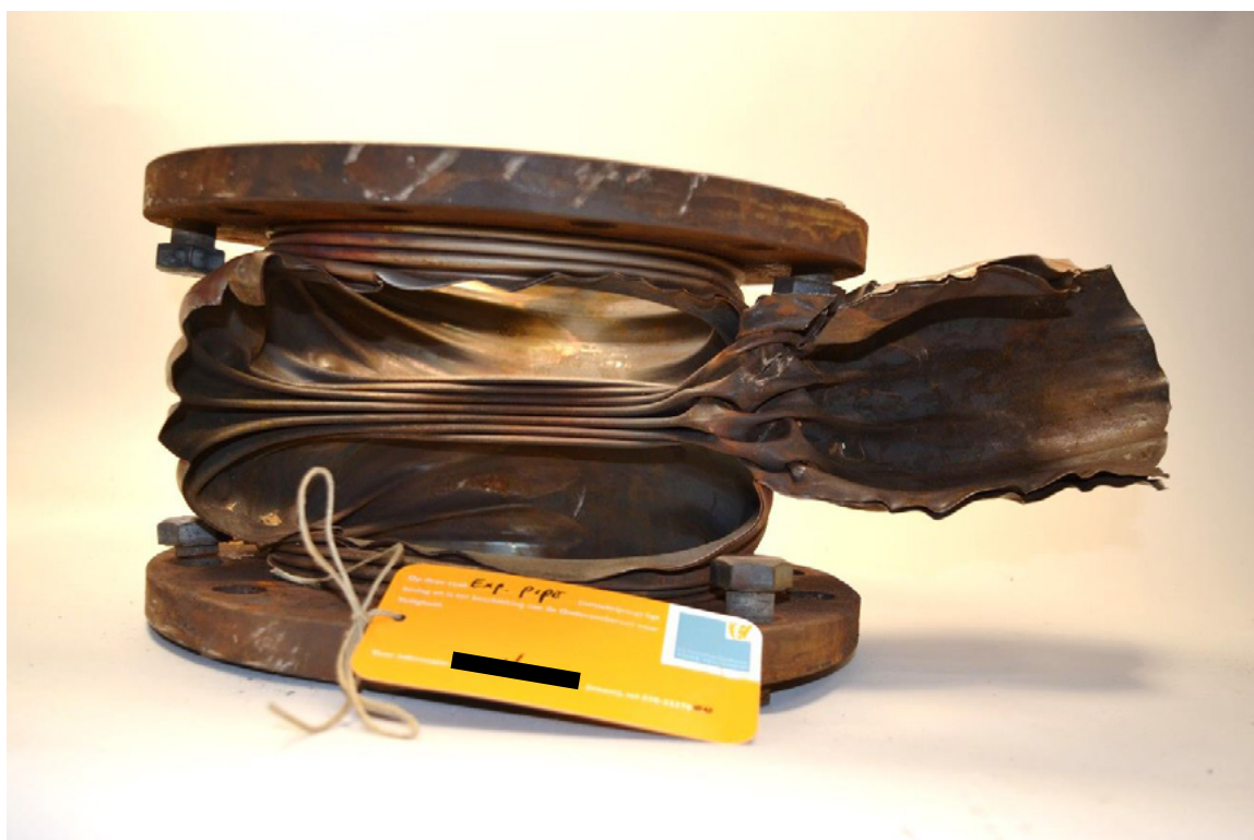
Figure 2. Overview of the fracture in the bellows with visibly expanded and compressed convolutions, the fractured double plate segment is still connected to the bellows.
