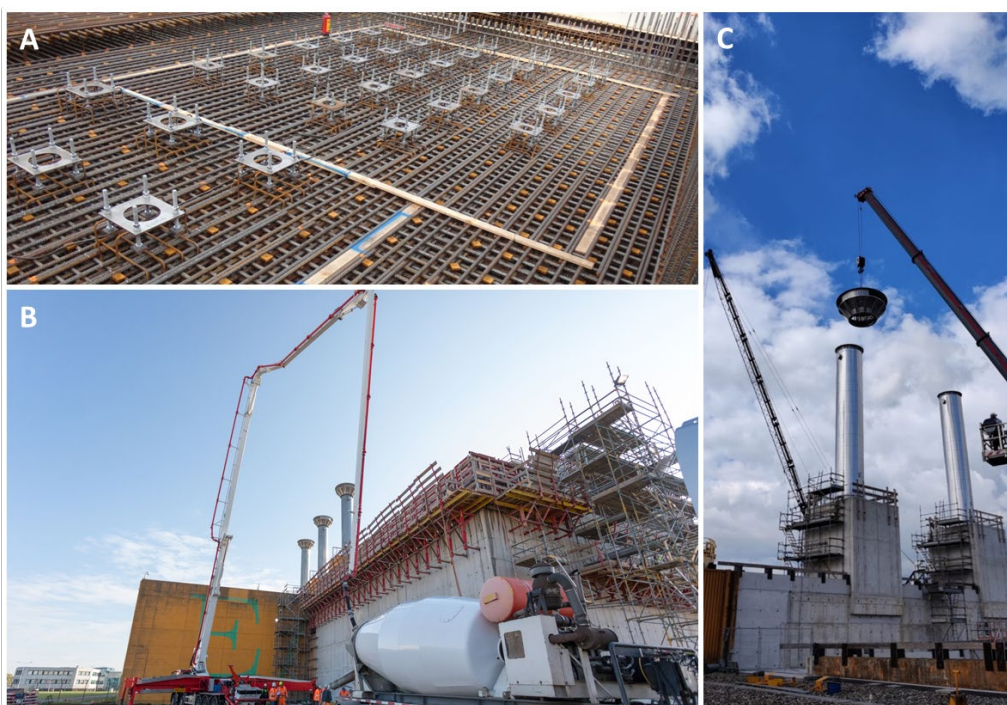
Figure 5.5: Construction on the extension of HABOG. A. heavy reinforcement in the concrete floor on which the wells are placed. B. Pouring concrete for 1,7 m outer walls. C. with the emplacement of the ventilation shafts the construction reaches its highest point.
